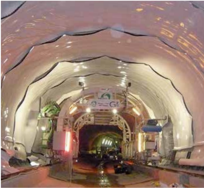
Tunnel, PVC 0.1 inch (2.5 mm)
